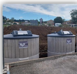
Conteneur semi enterré
